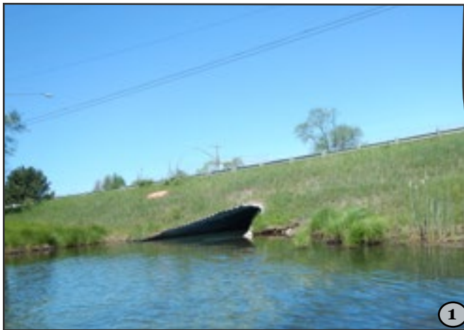
1. Undersized culverts can result in impounding of water.
